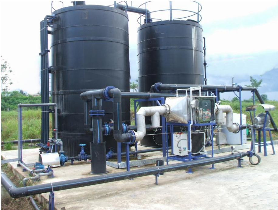
A BKE 400 m 3 /h Biogas Dryer (BD400) @ Sarawak, Malaysia
